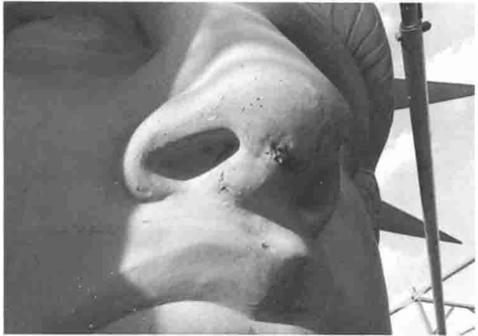
Fig. 11 Moisture that collected on the inside of the Statue of Liberty caused galvanic corrosion of the iron armature in contact with the copper skin. The copper skin on the nose was ruptured due to mechanical forces of the resulting corrosion products. Courtesy of R. Baboian, Texas Instruments, Inc.
