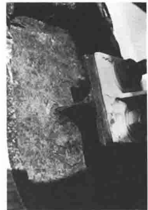
Fig. 7 Heavy corrosion of a steel support bracket where it passed through cellular glass insulation on a cold-temperature column. Moisture condensed on the column shell where the support was warmed by the extended attachment.
