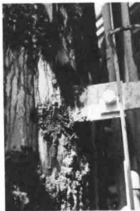
Fig. 8 Corrosion around the ladder clip of a gas-processing column. The column was painted with an inadequate protective coating (0.05 mm, or 2 mils, of epoxy) that could not prevent corrosion near the moisture entry points.
