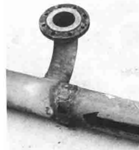
Fig. 9 Steel pipe corroded on the bottom side where a poorly sealed insulation joint allowed water to enter the insulation/pipe annulus. The moisture ran around the pipe and collected on the bottom.
