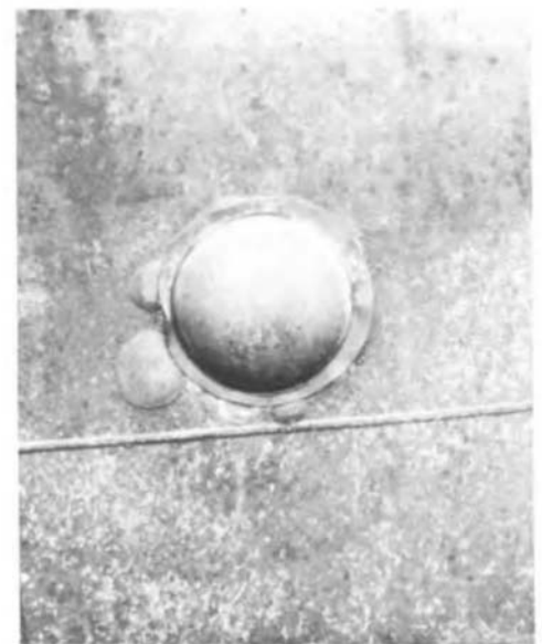
Fig. 12 Debonded organic coating near a high-silicon cast iron button anode
