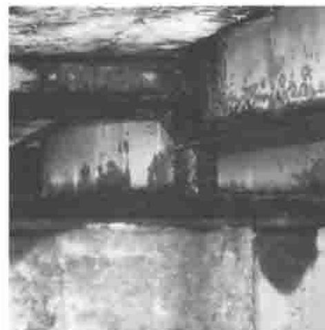
Fig. 5 Corroded regions on a painted highway bridge. Courtesy of R.H. Heidersbach, California Polytechnic State University
