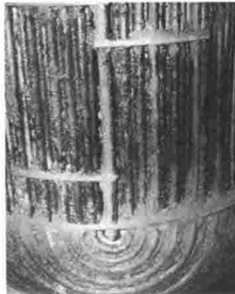
Fig. 5 Fouled heat-exchanger tube bundle
