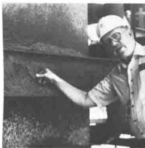
Fig. 6 Delamination of plain carbon steel due to \text{SO}_2 + ash deposit outside the boiler area of a coal-fired power plant. Courtesy of D.M. Berger, Gilbert/Commonwealth
