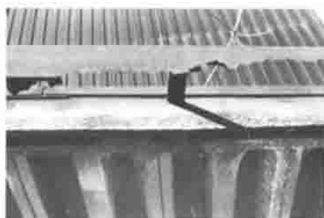
Fig. 3 Corroded weathering steel gutter. Courtesy of R.H. Heidersbach, California Polytechnic State University
